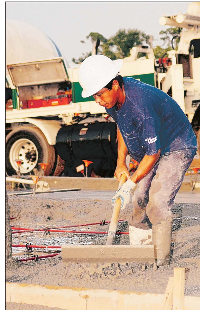
Photo by Kemberly Groue Above, contractor Apoliwar Zamora smooths a slab for a new home in Thrower Park, where walls went up Wednesday in for the first unit in the largest military family housing project in Air Force history. The $287.8 million program is building 1,028 new homes for Keesler families.
