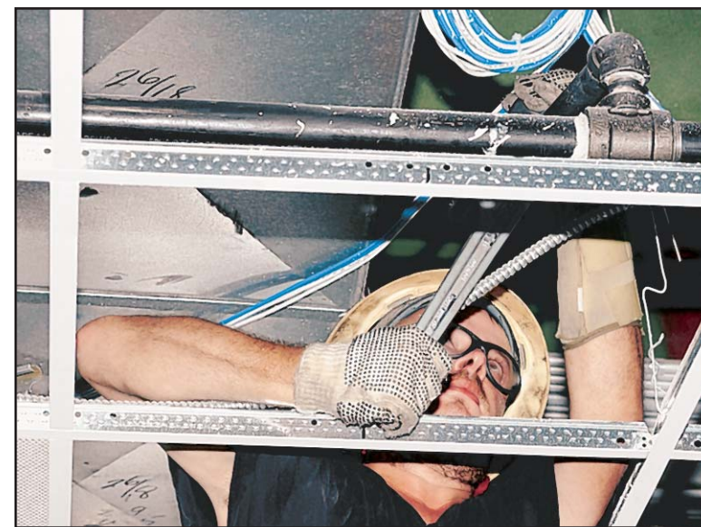
Below, contractor Bradley Hall adjust sprinkler heads inside the Sablich Center ceiling. The facility is scheduled to reopen in September.
