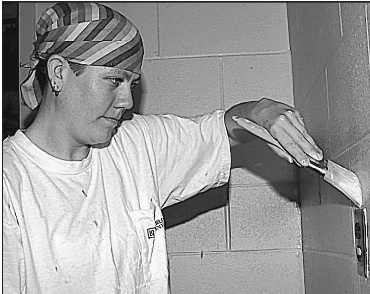
Photo by Kemberly Groue Jennifer Hudson from South Gulf Contractor of Florida paints the lobby area at Larcher Chapel.
