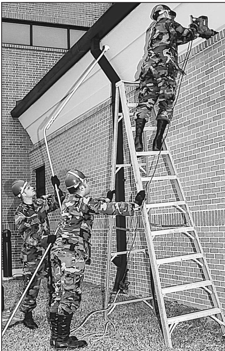
Airman Kiseleski holds an antenna while Sergeant Rodriguez steadies the ladder as Sergeant Hunt drills a hole for mounting the antenna outside Cody Hall Feb. 14. They're members of the 85th EIS.
