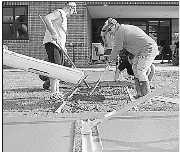
Tech. Sgt. Ryan Johnson, left, Capt. Jerry Bennett and Master Sgt. Robert Mayer, 45th Airlift Squadron, smooth out the cement for a walkway and barbecue grill pad behind Lott Hall.
