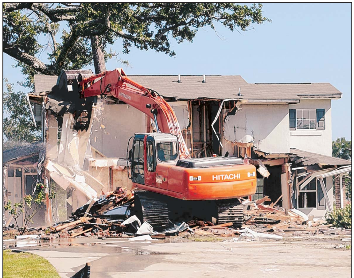
Rick Lacla, an excavator operator from Milam Construction of El Dorado, Ark., levels a home in South Pinehaven Aug. 18 that was ravaged by Hurricane Katrina's storm surge.
