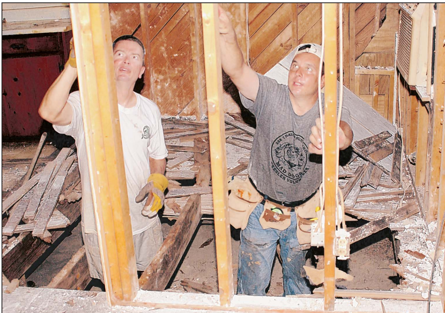
Maj. Matt O'Donnell, left, and Master Sgt. Dean Ross, 332nd TRS, pull up rotted flooring and remove nails from framing of the Schuler home. The home received extensive hurricane damage.
