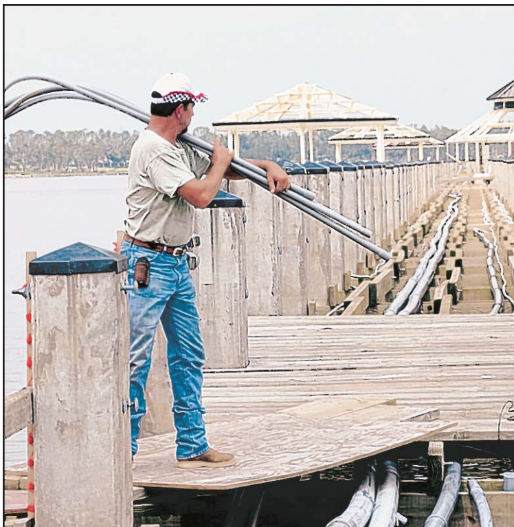
Contractor Tommy Hendrix prepares to carry a load of electrical conduit down the pier for installation.
