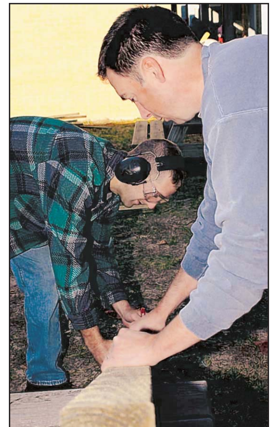
Tech. Sgt. David Hollyman, left, and Senior Master Sgt. Jim McClish measure a piece of lumber to be used to build benches inside the courtyard at Beauvoir Elementary School. They're from the 81st Transportation/Supply Squadron.
