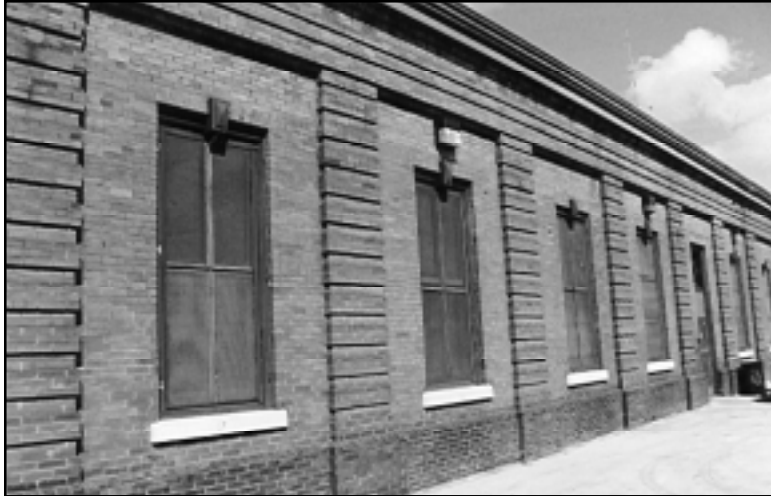
Figure 84. Drainage Pumping Station No. 1. View of east facade, showing brick depth and projection.
