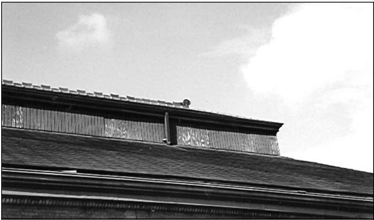
Figure 92. Drainage Pumping Station No. 1. View of the monitor roof peak at the northern end of the building, with terra-cotta crest and finial.
