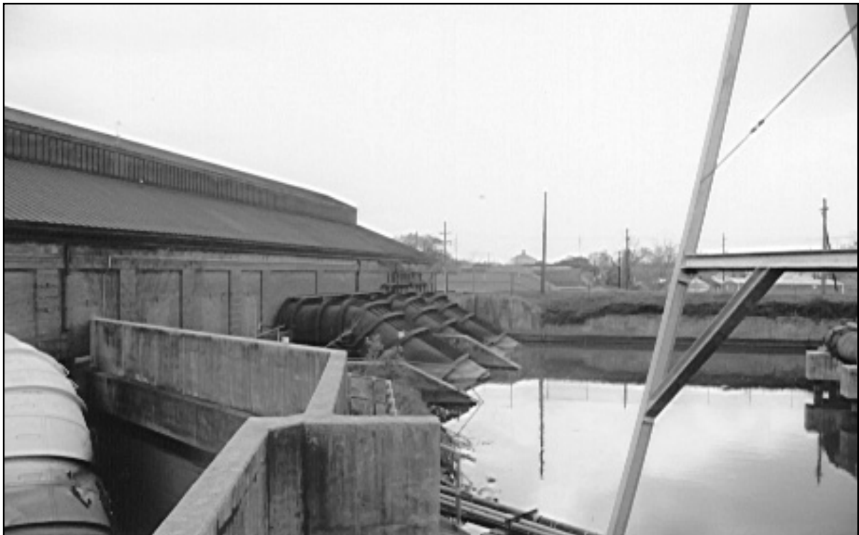
Figure 44. Drainage Pumping Station No. 3. View of discharge basin; 12' Wood pump at left, 14' Wood pumps at right (west) end of the station.
