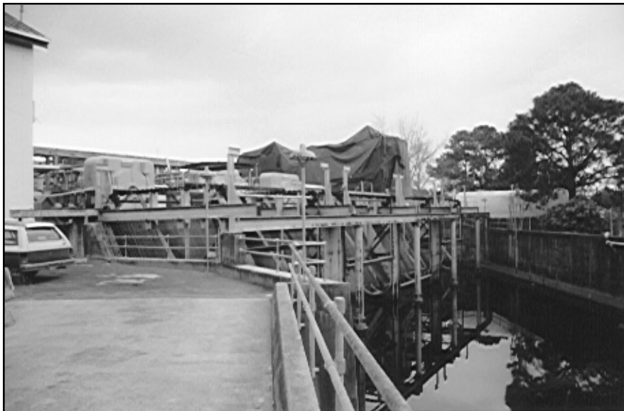
Figure 48. Drainage Pumping Station No. 4, viewed from the southeast. Pumping equipment is obscured by a tarpaulin; sand-blasting in progress.
