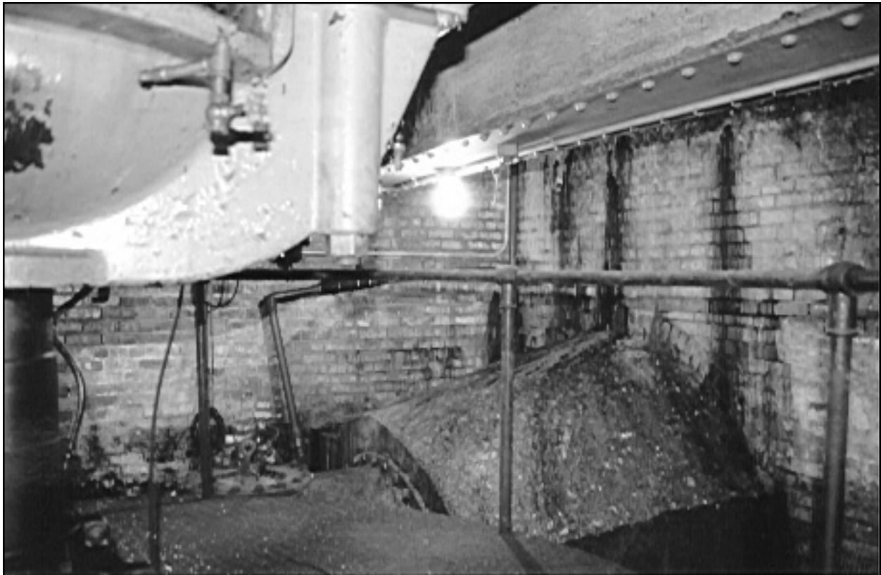
Figure 20. Vertical centrifugal pump pit, showing top of discharge pipe at right. These original pump pits, dating to 1897-1903, have been altered or eliminated at all stations except at Drainage Pumping Station No. 7, shown here.
