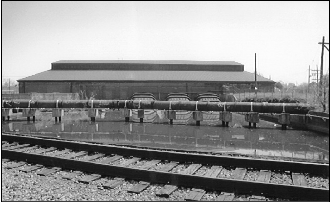
Figure 45. Drainage Pumping Station No. 3, viewed from railroad bridge over the London Avenue Outfall Canal. View of the discharge basin.
