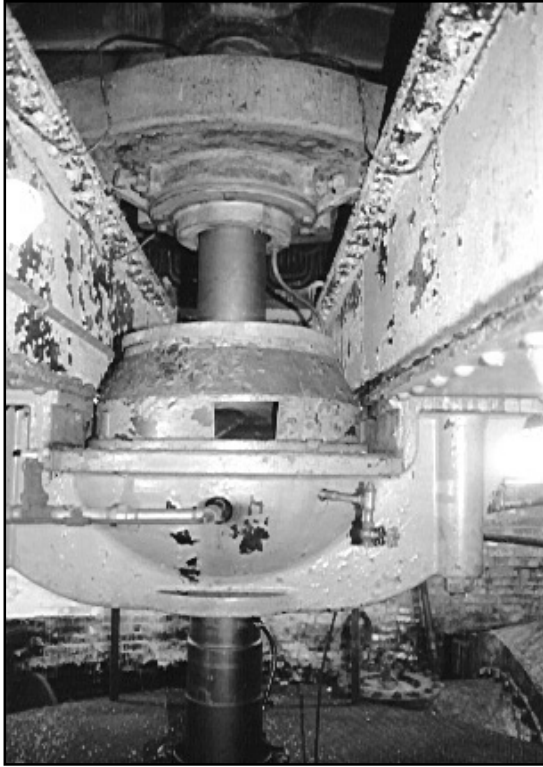
Figure 19. Lower portion of vertical centrifugal pump motor and drive shaft, of the type originally installed in Drainage Pumping Stations Nos. 1, 6, and 7, 1897-1903. Photographed at Drainage Pumping Station No. 7.
