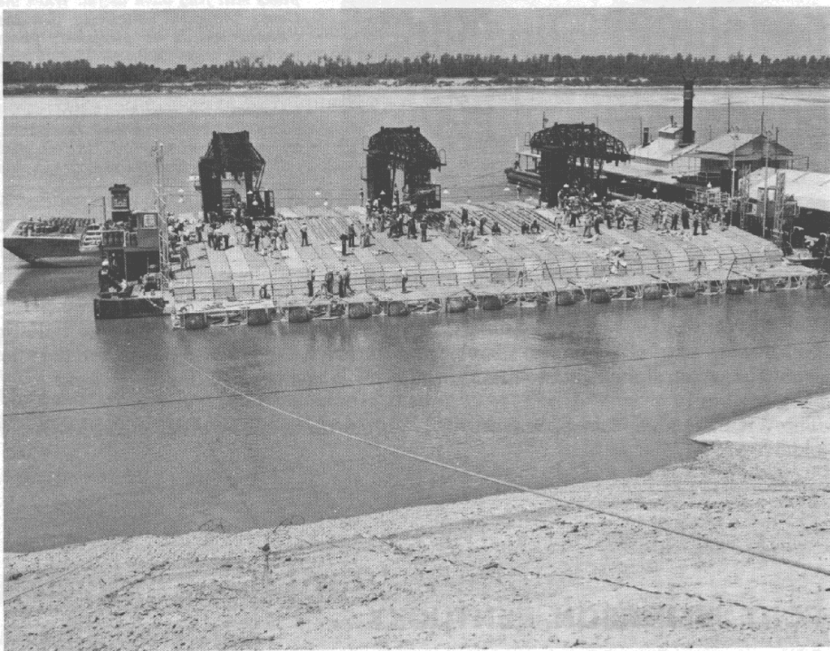
MAT-SINKING UNIT AT WORK. The mat-sinking unit shown in the above photo is in the process of laying an articulated concrete mattress designed to stabilize the river bank at the work site. The mattress, which consists of huge concrete blocks, is assembled at the site and lowered into place from a barge designed especially for this work. The fleet maintained and operated by the Army Corps of Engineers contains several of these mat-sinking barges.
