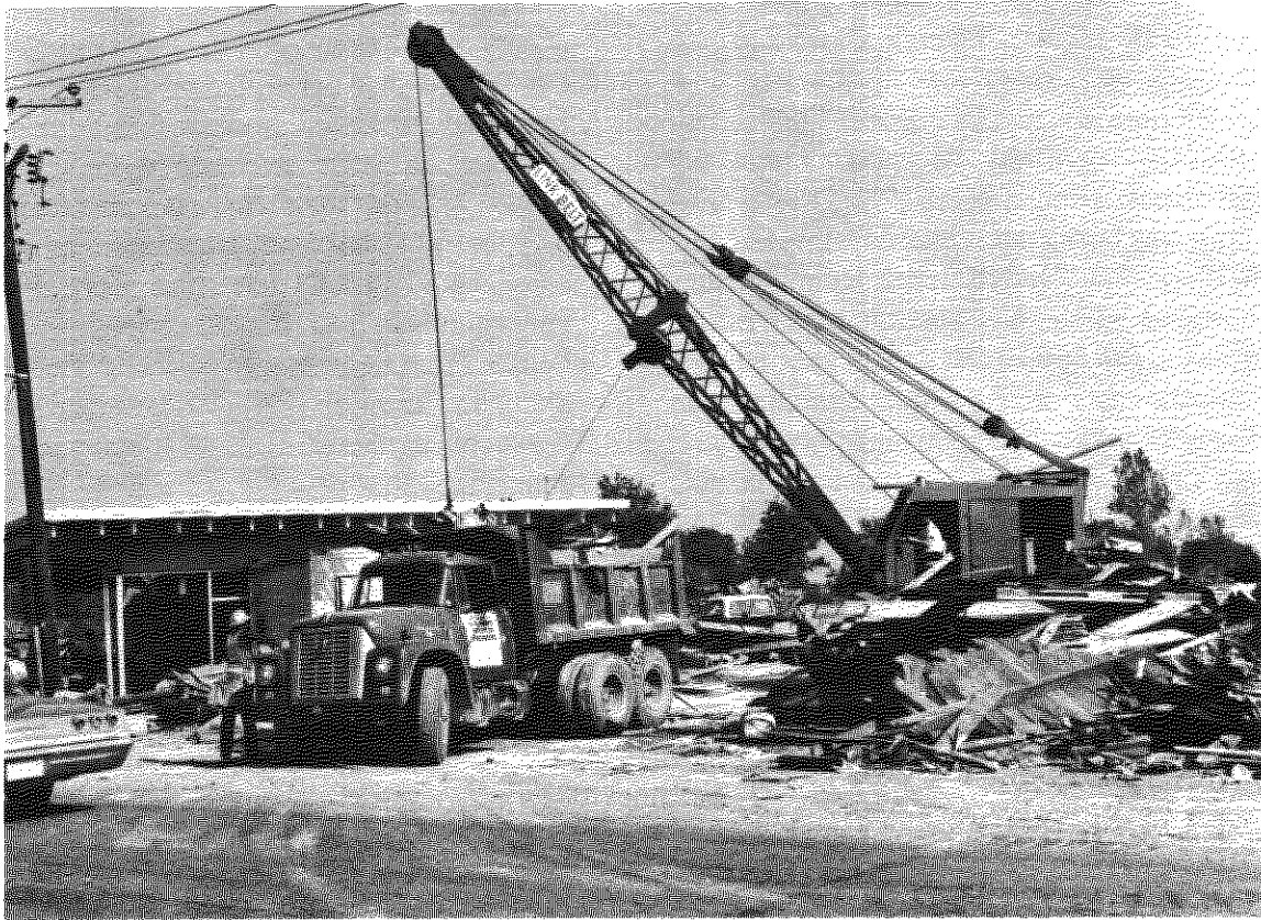
Hurricane damage cleanup.
