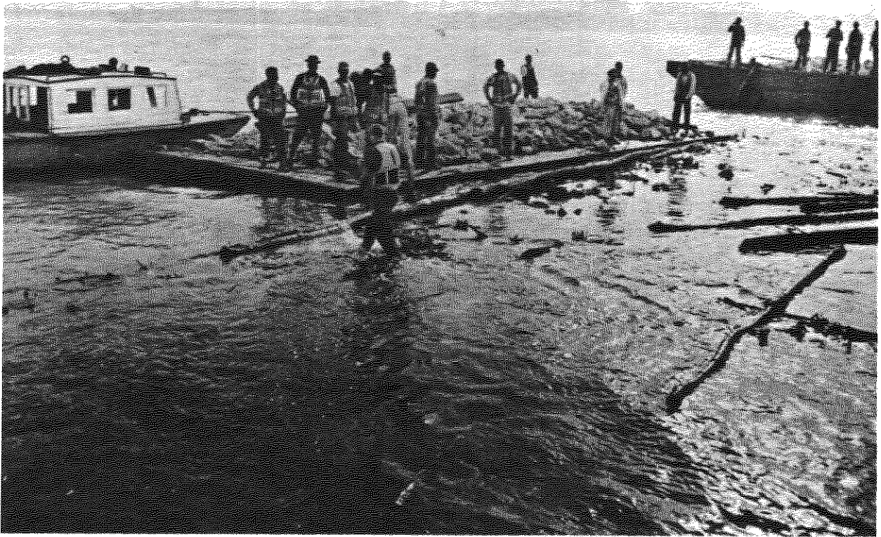
"Walking on the Water." Evenly distributed crushed rock gradually sinks a willow mat beneath the water. (Photo by C. Fortier)
