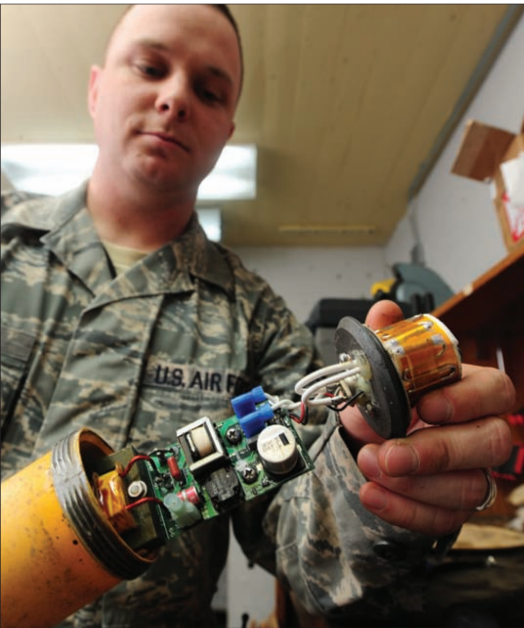
Staff Sgt. Clint Smith, 509th Civil Engineer Squadron electrical systems craftsman, repairs an inoperable taxiway edge light, Jan. 29. Taxiway edge lights are used to assist aircraft as they land and takeoff the runway at night and during adverse weather conditions.
