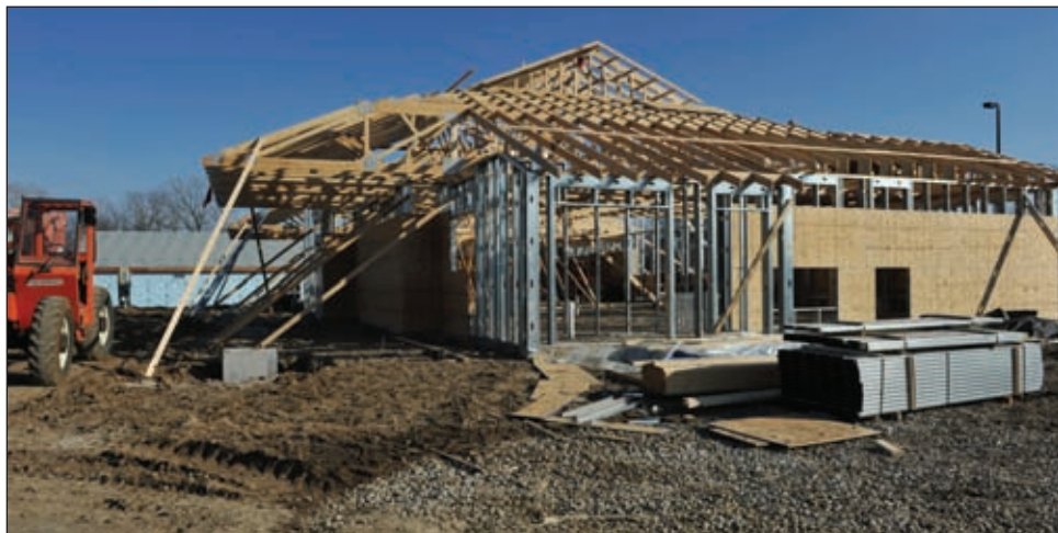
Balfour Beatty Communities construction workers build on the foundation for a new community management office, Jan. 22. The new facility will have several offices, a conference room and a room for greeting residents.
