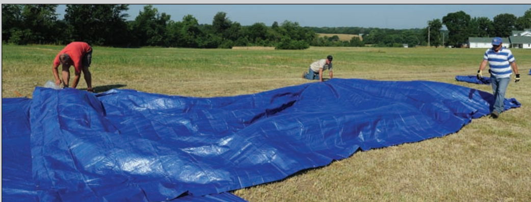
SEDALIA, Mo. -- Brian Kohrs, and Rick Lutz, Green Deconstruction Company construction workers, and Brian Bouy, J&B Builders construction worker, lay out a tarp as the projected landing spot for a cell tower demolition June 28. Repeater towers are signal amplifiers used to boost cell phone reception in the local area.
