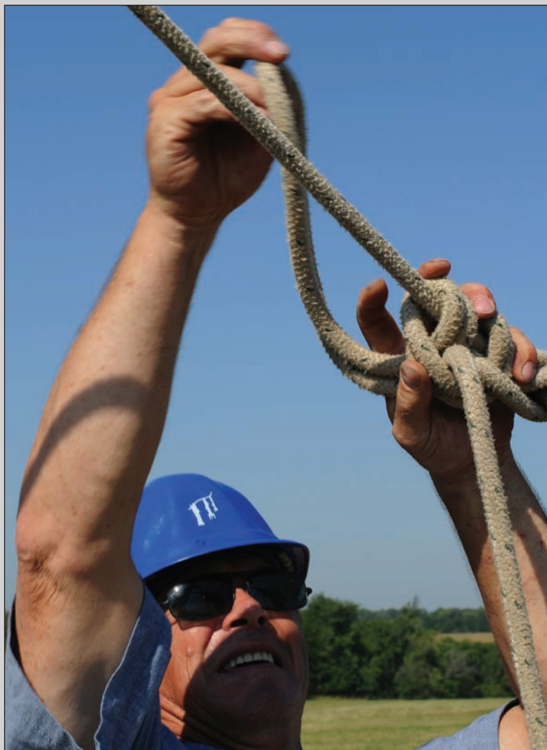
SEDALIA, Mo. -- Robert Camp, ALT Inc. construction worker, ties a rope before bringing down an Air Force cell tower June 28. The tower was demolished because it was no longer in use.
