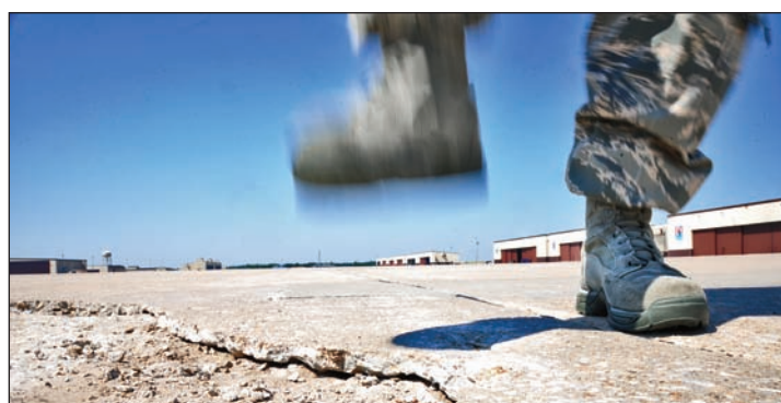
An Airman from the 509th Operations Support Squadron airfield management operations flight stomps on cracked pavement to check solidity as part of a routine flight inspection June 29.
