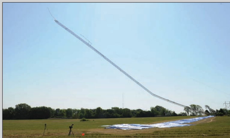
SEDALIA, Mo. -- A 416-foot cell tower, property of the U.S. Air Force, came crashing down June 28. The 509th Civil Engineer Squadron contracted J&B Builders to complete the demolition.
