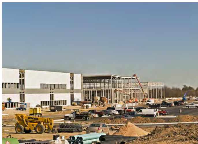
Construction of the LG Chem 850,000-square-foot lithium-ion polymer battery cell and battery manufacturing facility is taking place in Holland, Michigan. LG Chem is a key supplier of batteries to General Motors for the Volt Program.
