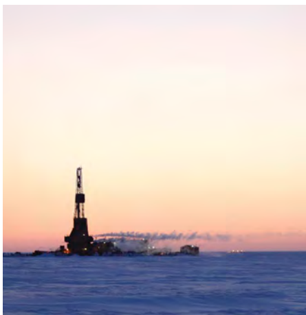
The landmark Mt. Elbert gas hydrate field evaluation program is headquartered at the Mt. Elbert well on the Alaskan North Slope.
