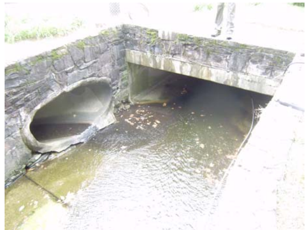
Figure 2: Culvert at upstream limit of underground portion of the unnamed tributary before flowing behind the homes on Brookside Road.
