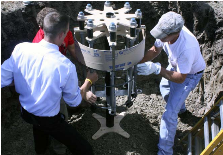
A team sets the SMART Foundation in place before the concrete pour for the Wind for Schools project installation at Eudora High School in Eudora, Kansas. Photo from Kansas State University, NREL/PIX 19692
