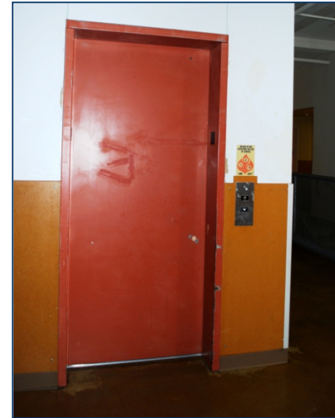
Elevator to second floor at emergency shelter
