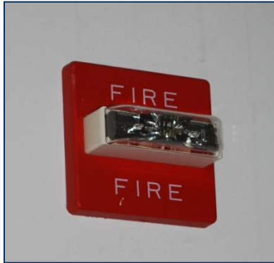
Fire alarms with strobe lighting
