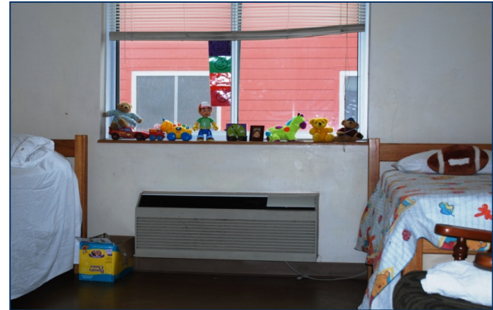
Individually-controlled air- conditioner unit in emergency shelter bedroom
