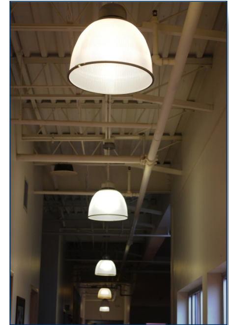
Incandescent hallway lighting
