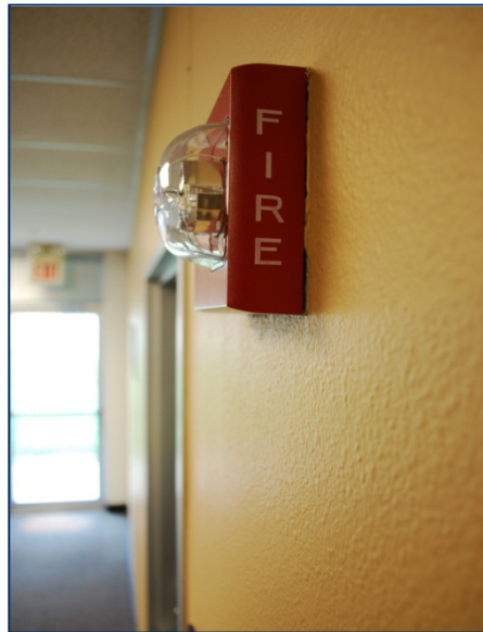
Fire alarm with strobe lights
