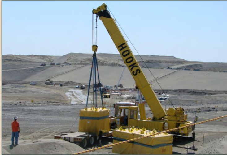
Offloading Ion Exchange Module in ERDF
