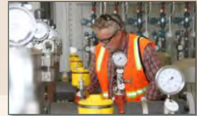
Optimizing water treatment
