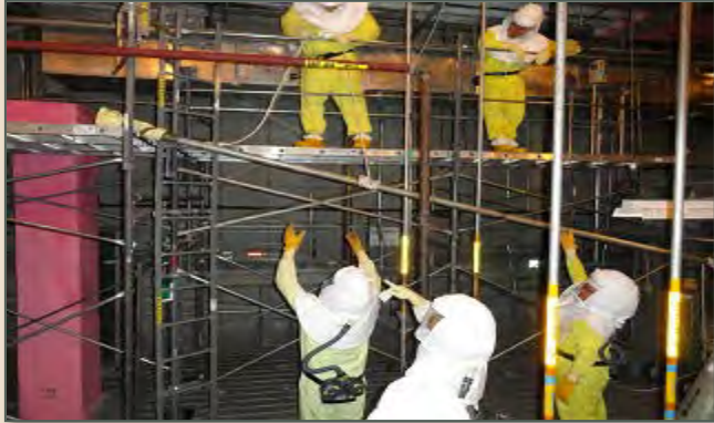
Photos of the Process Vacuum Piping Removal in Room 262 in the duct level
