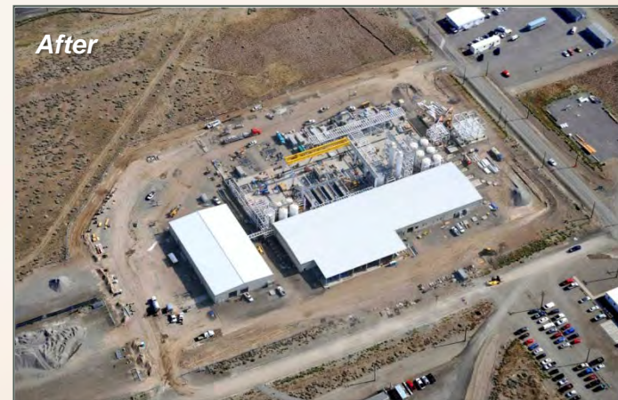
200 West Pump and Treat System
