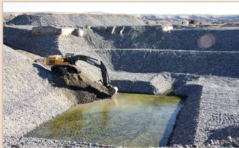
Removed more than 150,000 tons of waste material and chrome contamination from 100-F-57 waste site.
