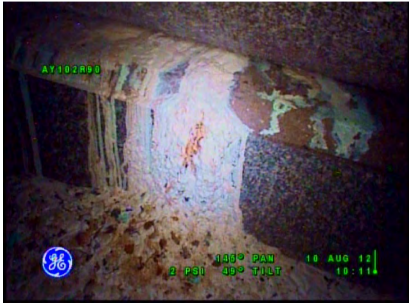
White material on top of refractory and along edge of curb
