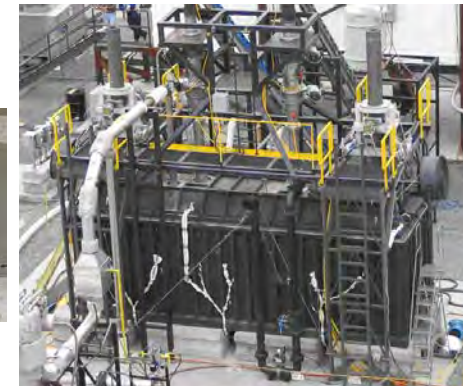
Bulk Vitrification - Joule heated melting in a refractory lined steel box
