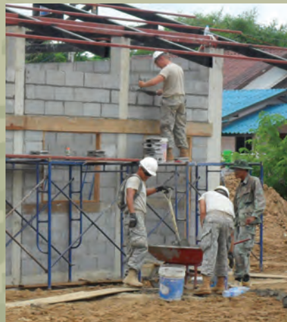
Members of the 646 th Contingency Contracting Team, Taegu, South Korea, provided cradle-to-grave contracting support to the 643 rd Engineering Company, the 84 th Engineering Battalion and the Washington Army National Guard Special Operations Detachment–Pacific, from May 22 through July 1 during Ayara Guardian 2011, a training exercise in Thailand. The team was in the Pran Buri District to fully support each unit’s training requirements for partner nations’ combined engineering civic action projects and command and control/engineering assistance responsibilities and their execution.
