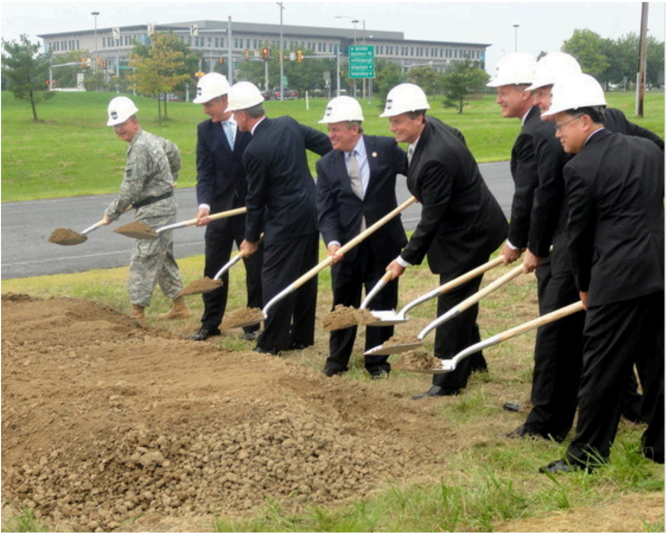
Officials break ground on the 43,000 square-foot post, Friday, August 17, 2012. Sen. Bob Casey, Reps. Tim Murphy, Mike Doyle, Jason Altmire and Mark Critz, and Allegheny County Executive Rich Fitzgerald each spoke at the ceremony.
