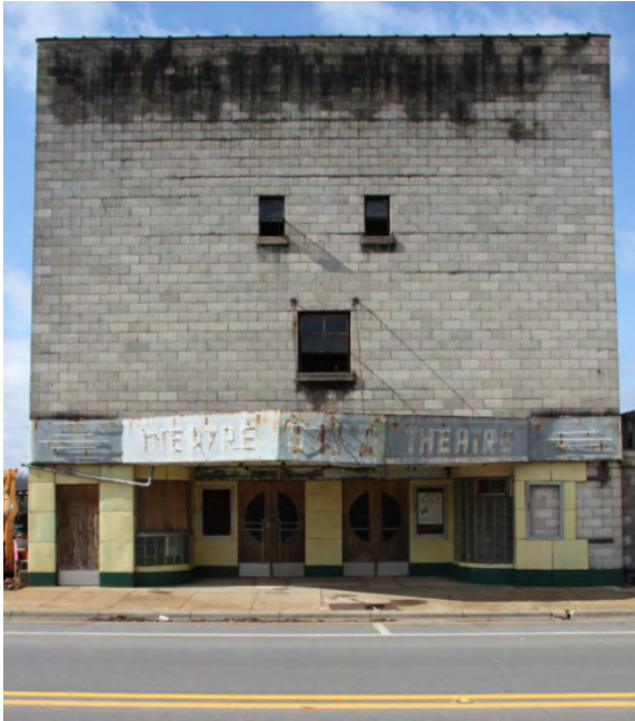
Figure 4-94: The historic Star Theatre in downtown Moulton is being considered for redevelopment.
