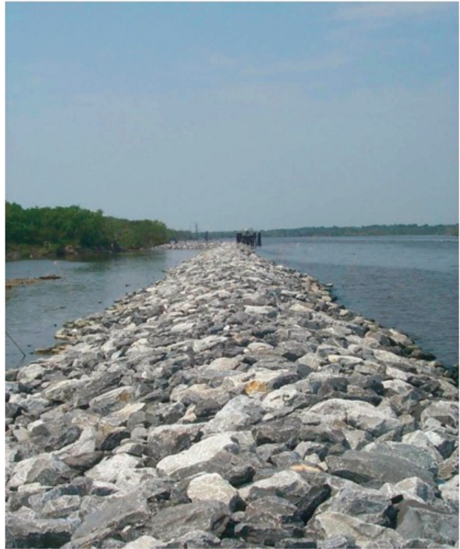
Protection will be provided to a total of 41,000 feet of shoreline in order to preserve the effectiveness of these areas in preventing marsh loss.
