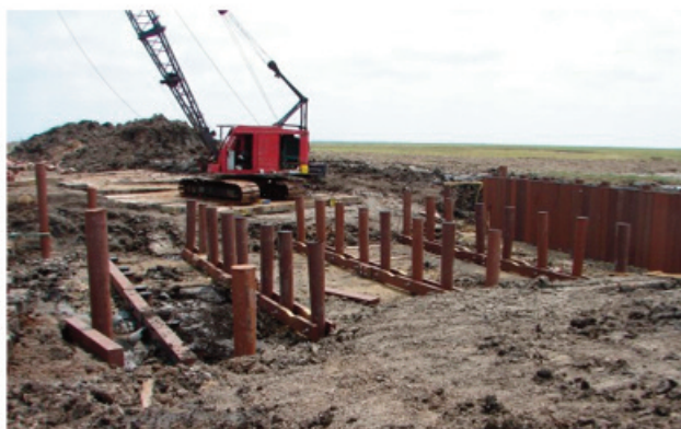
Early stages of the construction of a water control structure to move freshwater to brackish marshes to the south.
