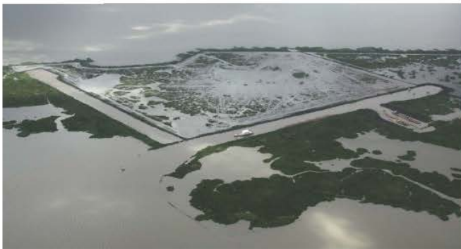
Aerial view of the east end of Marsh Island after commencement of construction activity.
