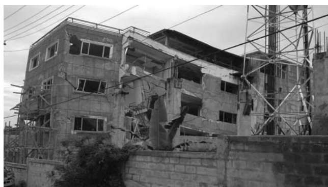
Figure 4. Damage to a recently constructed commercial building approximately 0.5 km west of HVCV. The building was later demolished.
