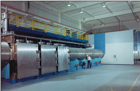
The Uranium Demonstration System at LLNL tests the AVLIS process at plant scale.
