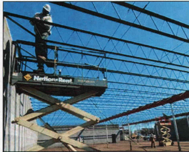
This workman in repairing the remaining roof supports in preparation for the reconstruction of the dilapidated Longwood Plaza. This gut renovation was only "doable" because of the financial infusion from the sale of new markets tax credits.
