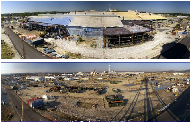
Accelerated Depreciation: Demolition of a metals fabrication plant at Fernald was completed in 2002.
