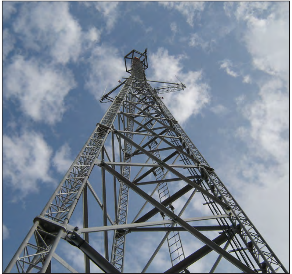
New communication tower at HARB: This new communication tower at Homestead ARB will improve the quality and security of radio transmissions at the base. The tower is the tallest structure at Homestead ARB, at over 200 feet tall (U.S. Air Force Reserve photo by Leo Castellano).
