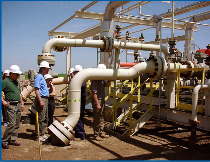
Weyburn-Midale is a commercial-scale project recognized by the Carbon Sequestration Leadership Forum that will utilize CO 2 for enhanced oil recovery. Photo of CO 2 pipeline as it enters Weyburn from Beulah, N.D., courtesy of Petroleum Technology Research Centre.
