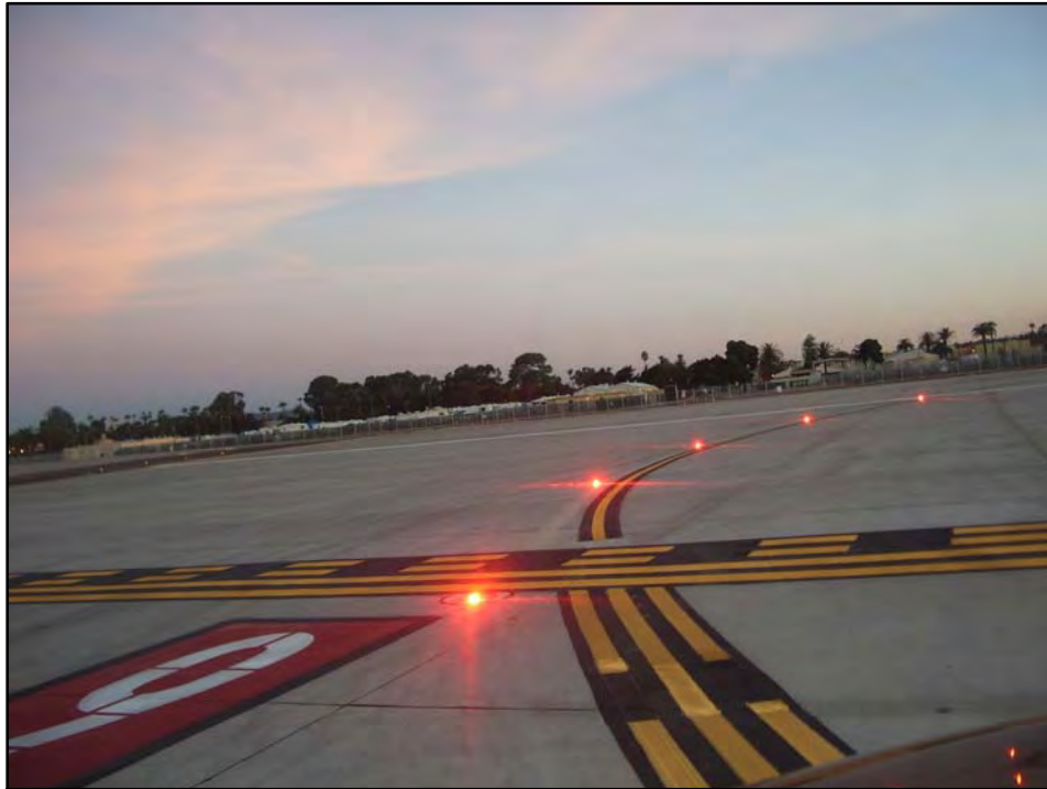
FIG AD 1.1-12 Runway Entrance Lights
