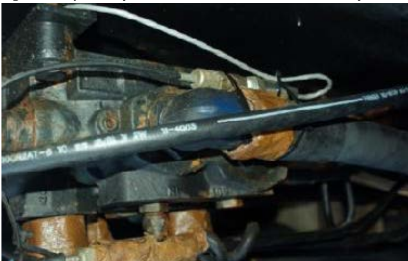
Figure A4 Hydraulic pressure transducer installed at trawl warp winch.
