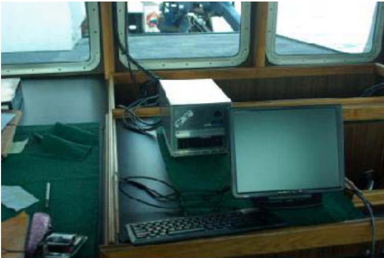
Figure A1. EM control box (V4) and user interface installation
