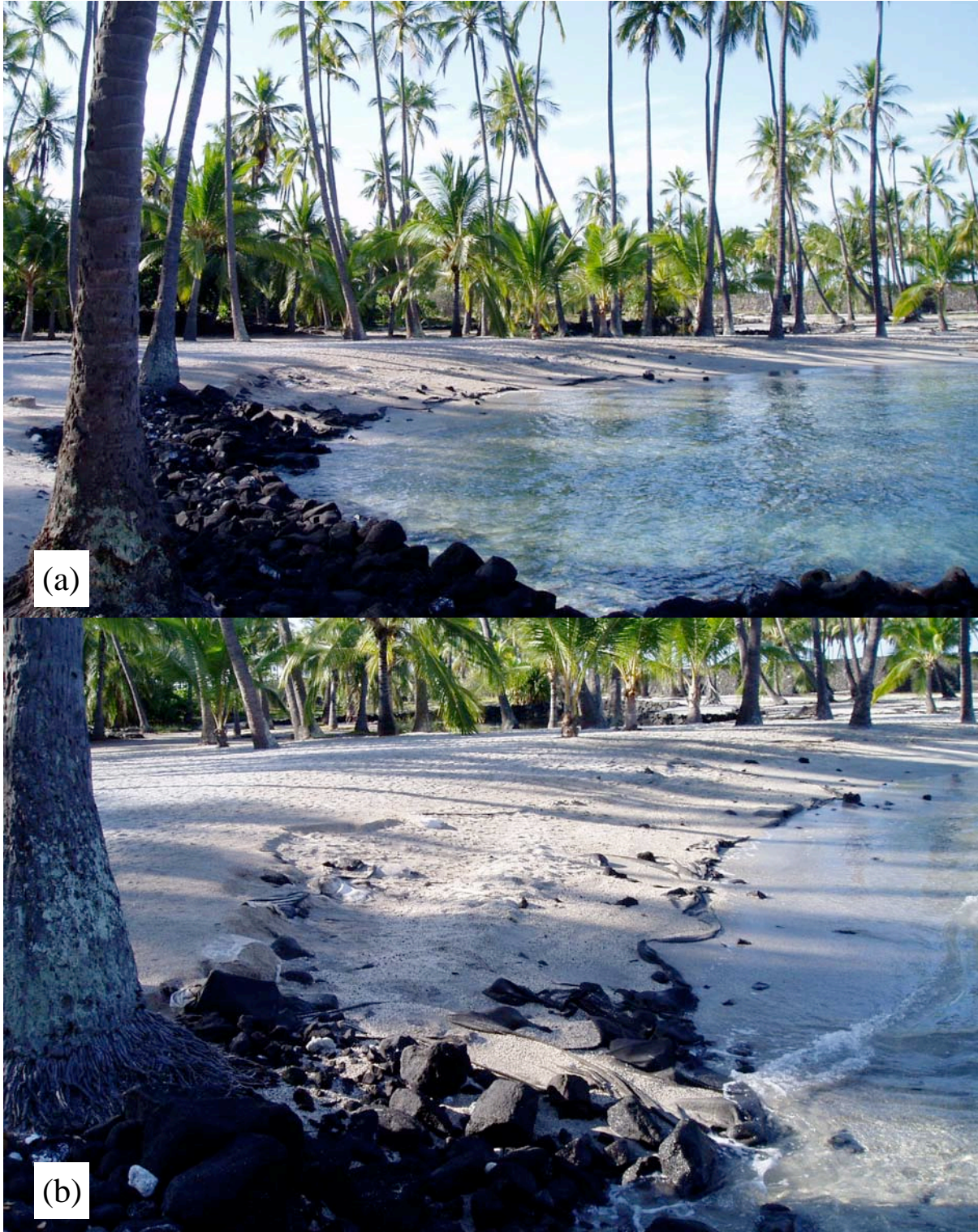
Figure 10. Erosion control fabric exposed along the head of Keone'ele Cove in December 2004. (a) View looking southwest from the east side of the cove. (b) Closeup of southeast corner of cove. Photos D. Hoover, 2004.
