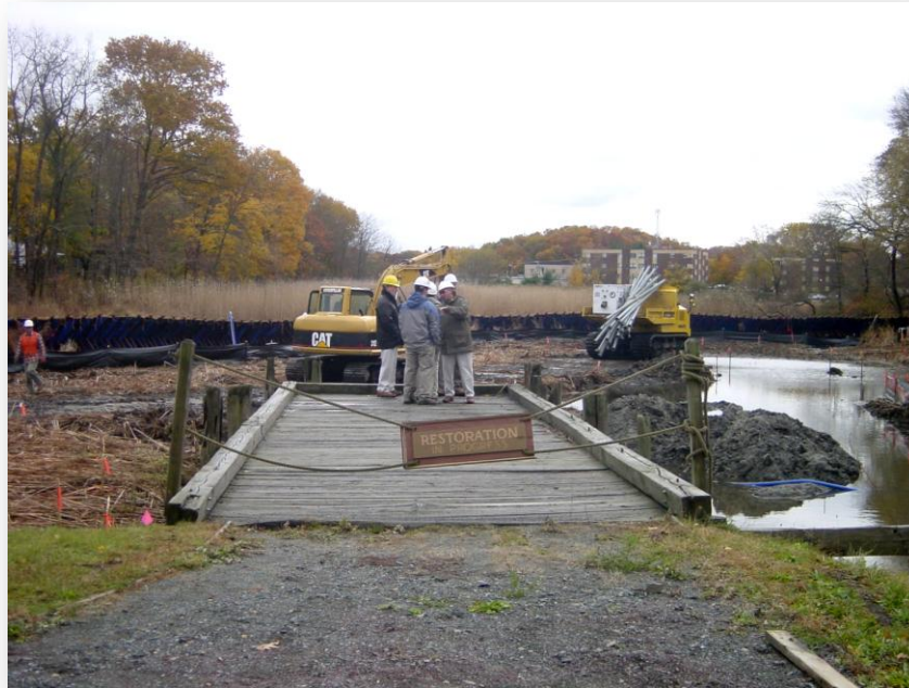
Figure 5. Phase I of the restoration (fall 2007): sediment excavation and creating open water in the turning basin. (Photo courtesy of MJ James-Pirri.)
