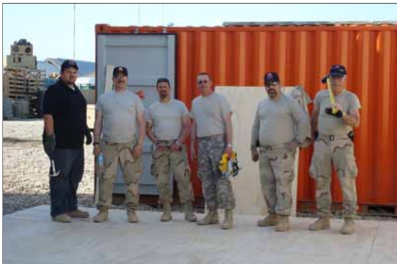
Members of the 1/10 MTN BLST admire their handiwork as they complete construction of the platform for the EELS tent.
