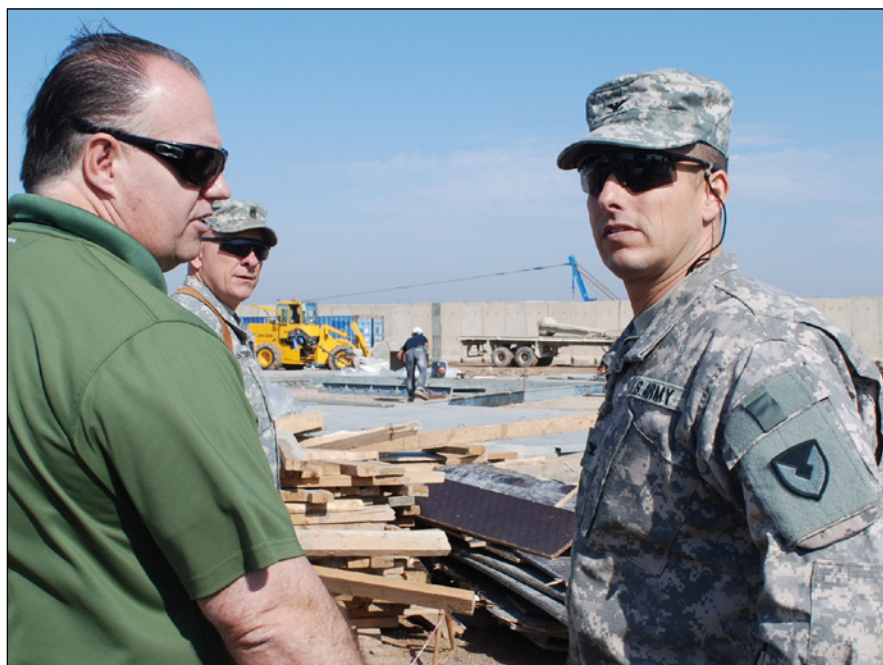
Col. John S. Laskodi, 402nd Army Field Support Brigade commander, discusses progress on the construction of a mine-resistant, ambush-protected vehicle maintenance facility at Basrah, Iraq, with Danna Buster, contracting officer's representative. The operation supports the State Department's continuing mission in Iraq.
