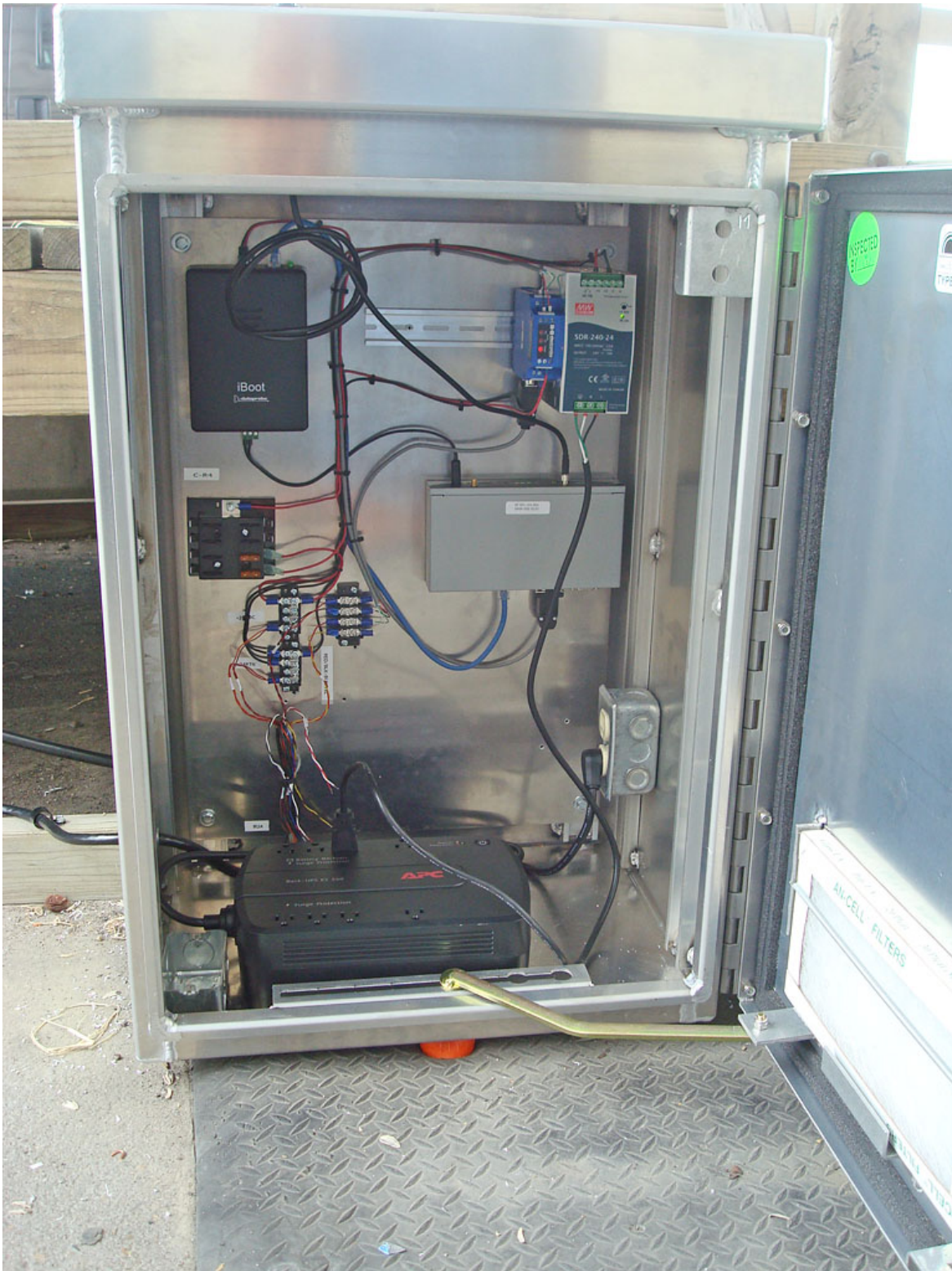
Exhibit 3. Representative Electronics Cabinet
