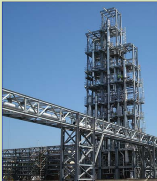
NCCC Post-Combustion Carbon Capture Center
