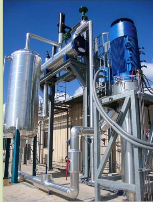
Liquid CO 2 Pump Loop Constructed at SwRI
