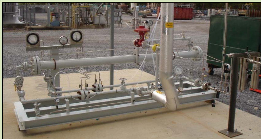
MTR Membrane Test Skid at the National Carbon Capture Center
