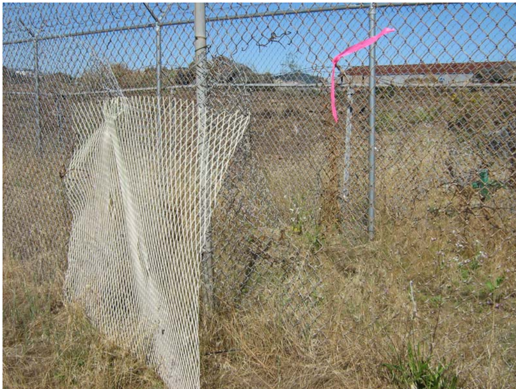
Breached section of northwest perimeter fence for Parcel E-2, June 30, 2011 quarterly inspection.
