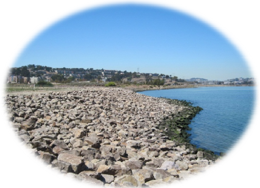
Parcel B Shoreline Armored with Large Rocks (Rip Rap)
