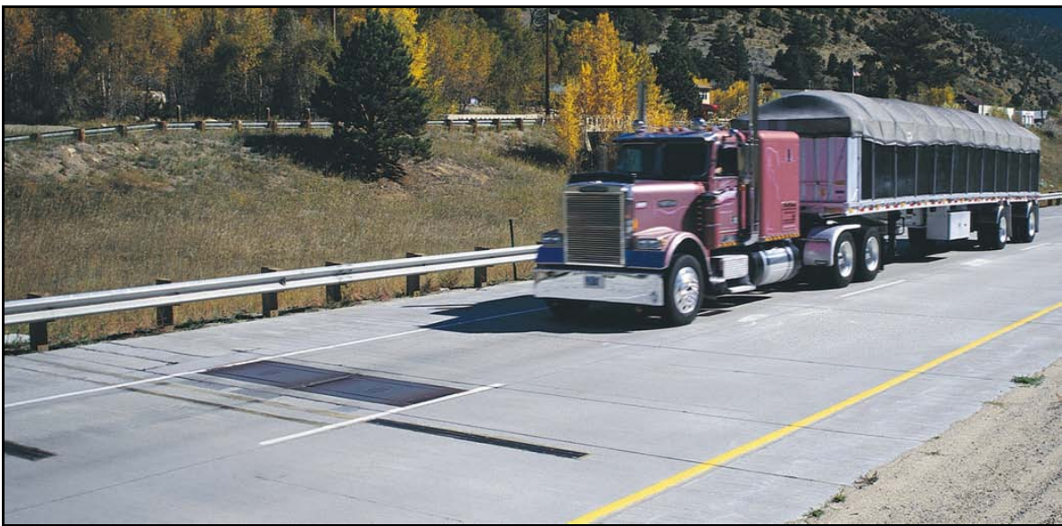
Figure 3. Photo. In-line weigh sensors (single load cells), a trailing axle sensor, and detection loops (single threshold system).
