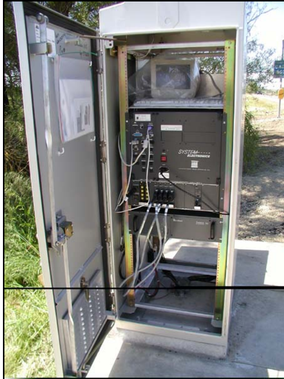
Figure 5. Photo. Controller cabinet, front view.
