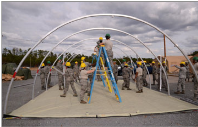
Members of the 94th Force Support Squadron erect a canopy during annual training at a Single Pallet Expeditionary Kitchen training site Dec. 5. (photo by Brad Fallin)
