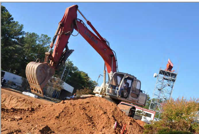
Contractors from Newkirk Electric dig at the site of a future Digital Air Surveillance Radar (DASR) Tower near building 557, Oct. 26. The tower, operated by the 94th Communications Squadron, will have digital capability, and will be more energy efficient. Completion of the tower construction is expected mid 2013. (photo by James Branch)
