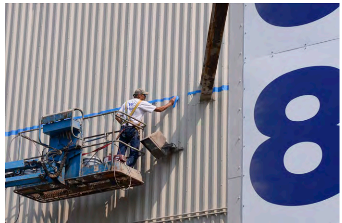
Contractors from Windamir Development and Construction repaint headquarters building 838 July 13. In addition, the $163,000 project consisted of power washing, sealing, and repainting exterior walls on buildings 486, 511, 513 and 514. (photo by Don Peek)
