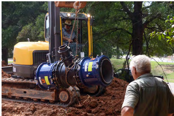
Personnel from SoCo Contracting Company (contractor for the 116th Air National Guard) install an 18 x 18 x six foot ductile iron tee to repair a water main leak on base July 19. (photo by Don Peek)
