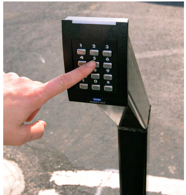
Keypads recently installed at base airfield entrance gates help increase security and accountability around Dobbins Air Reserve Base. (photo by Brad Fallin)
