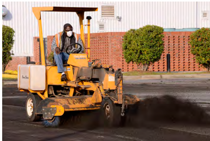
Base contractors sweep asphalt in preparation for repaving the parking lot at building 838, March 14. Various base locations received new parking surfaces this spring. (photo by Brad Fallin)
