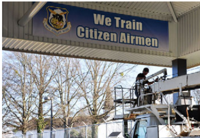
Contractors from Stone Co. Installation install banners in the entrance and exit lanes of the Dobbins entrance canopy Jan. 30. (photo by Senior Airman Danielle Campbell Purnell)
