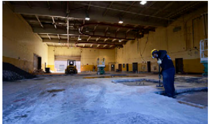
Contractors install new supports for an upper level structure and upgrade interior during construction in building 819 here Jan. 24. (photo by Don Peek)
